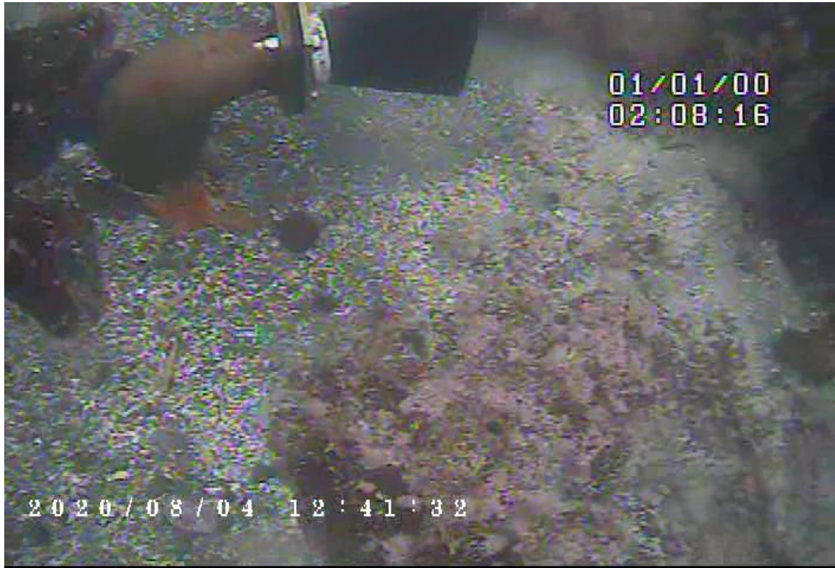
Photo 5 – Diffuser 11 showing strong flow
