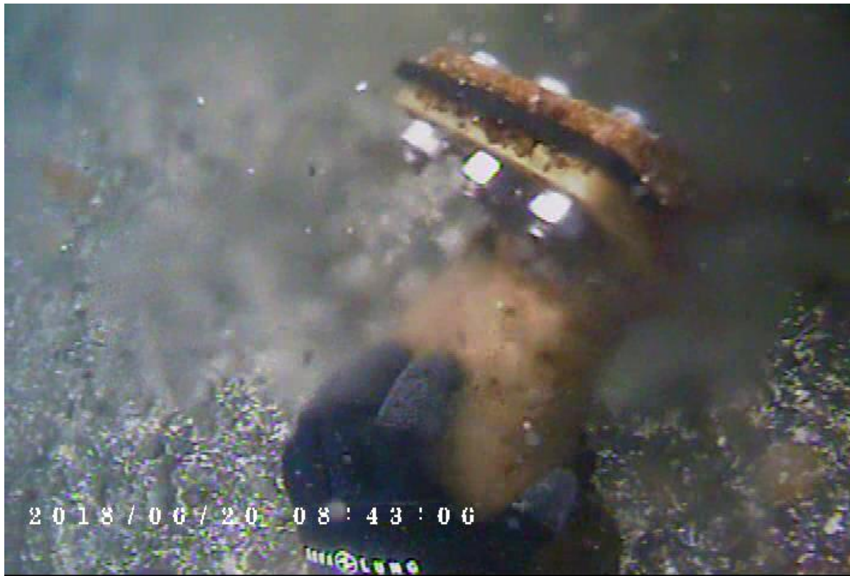
Photo 4 – Diffuser 4 showing strong flow
