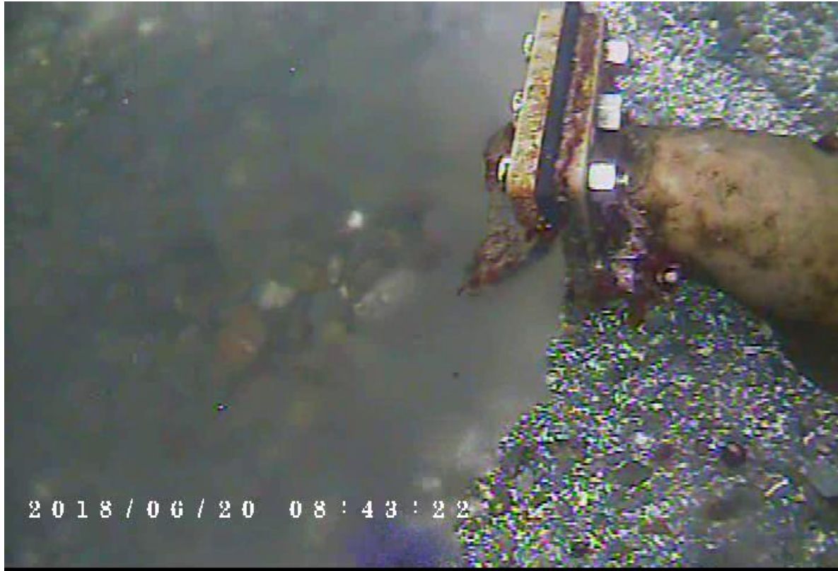
Photo 5 – Diffuser 5 showing strong flow
