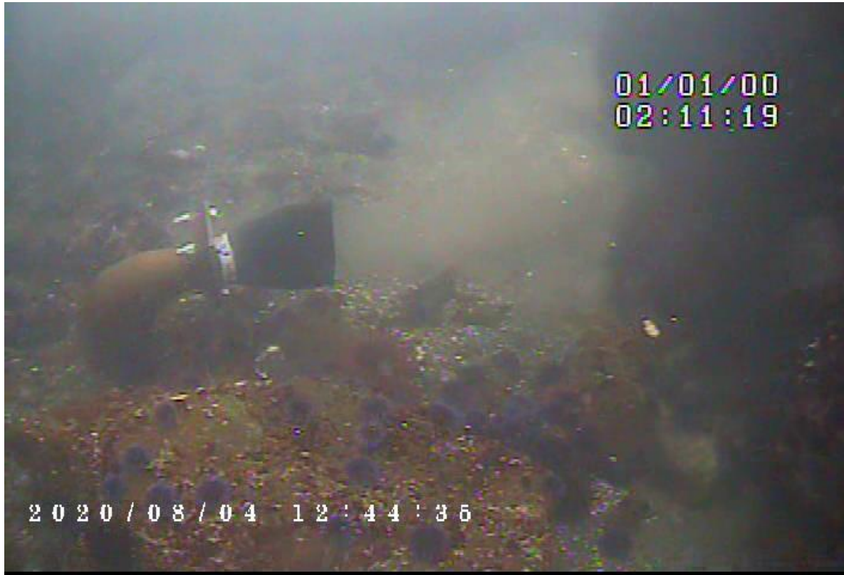
Photo 15 – Diffuser 1 showing strong flow
