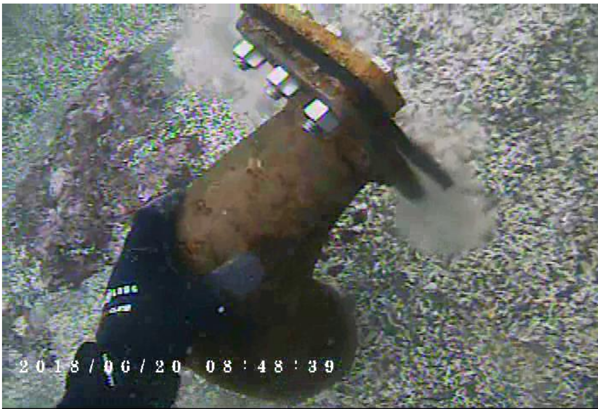
Photo 12 – Diffuser 12 showing light flow
