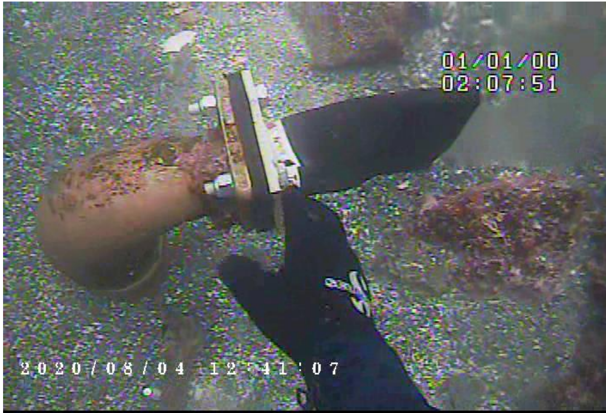
Photo 3 – Diffuser 13 showing strong flow
