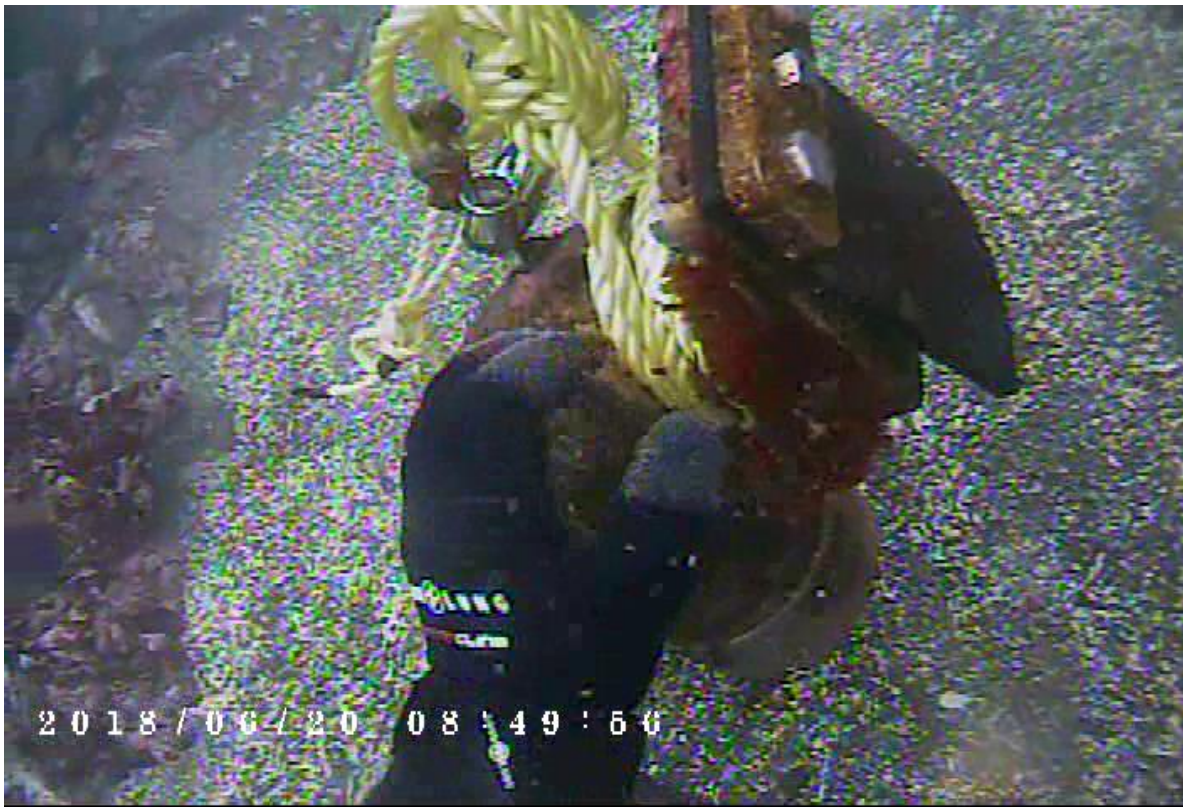
Photo 14 – Diffuser 14 showing no flow
