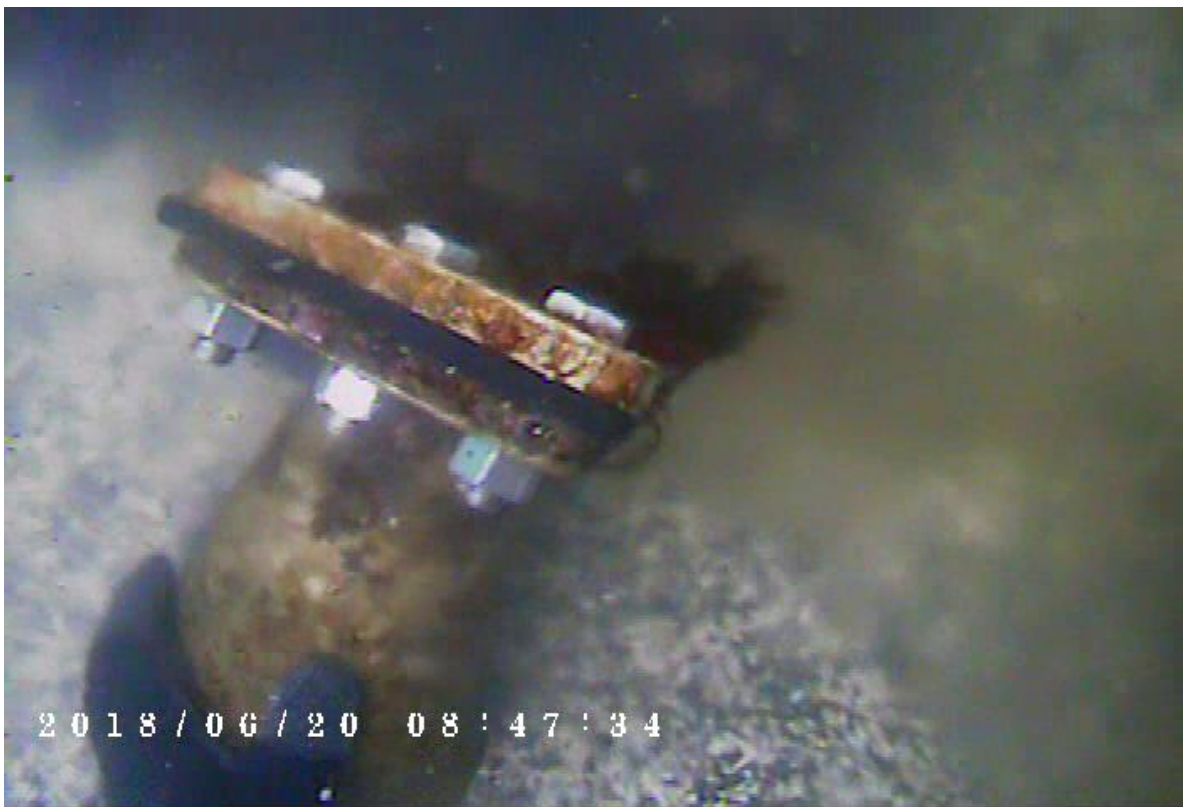
Photo 10 – Diffuser 10 showing strong flow
