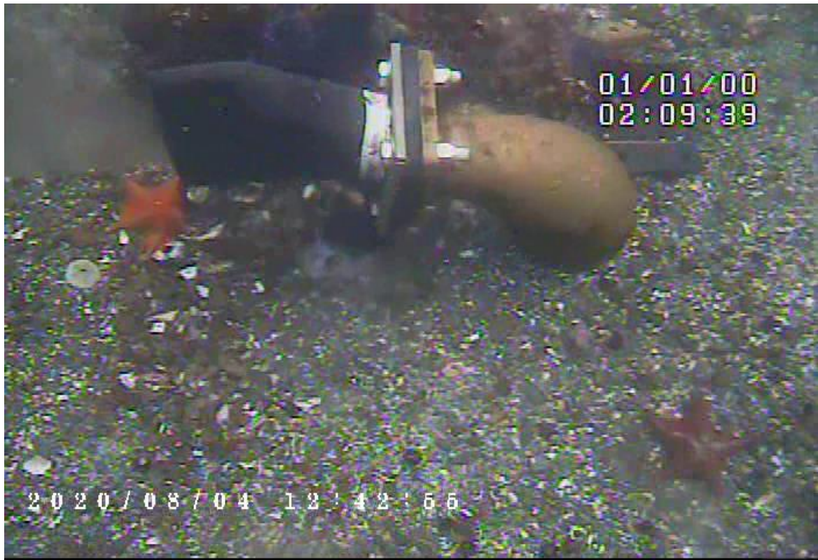
Photo 10 – Diffuser 6 showing strong flow
