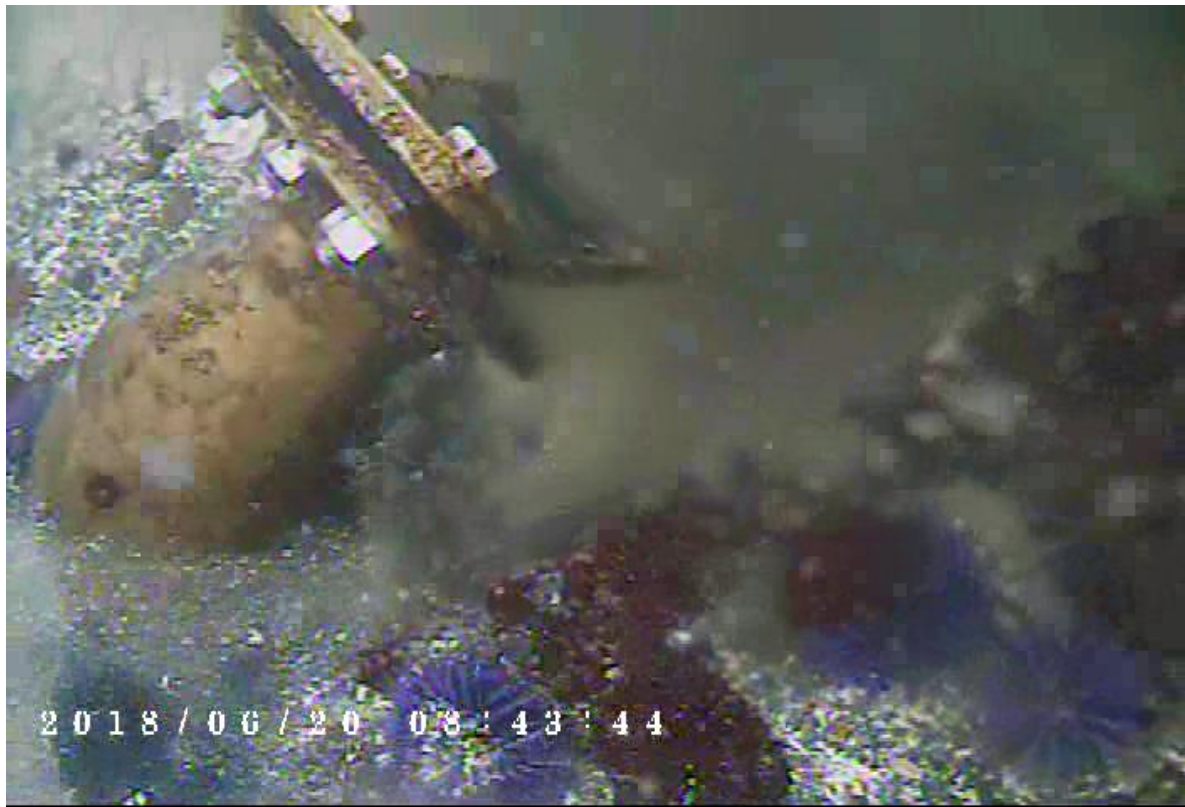
Photo 6 – Diffuser 6 showing strong flow
