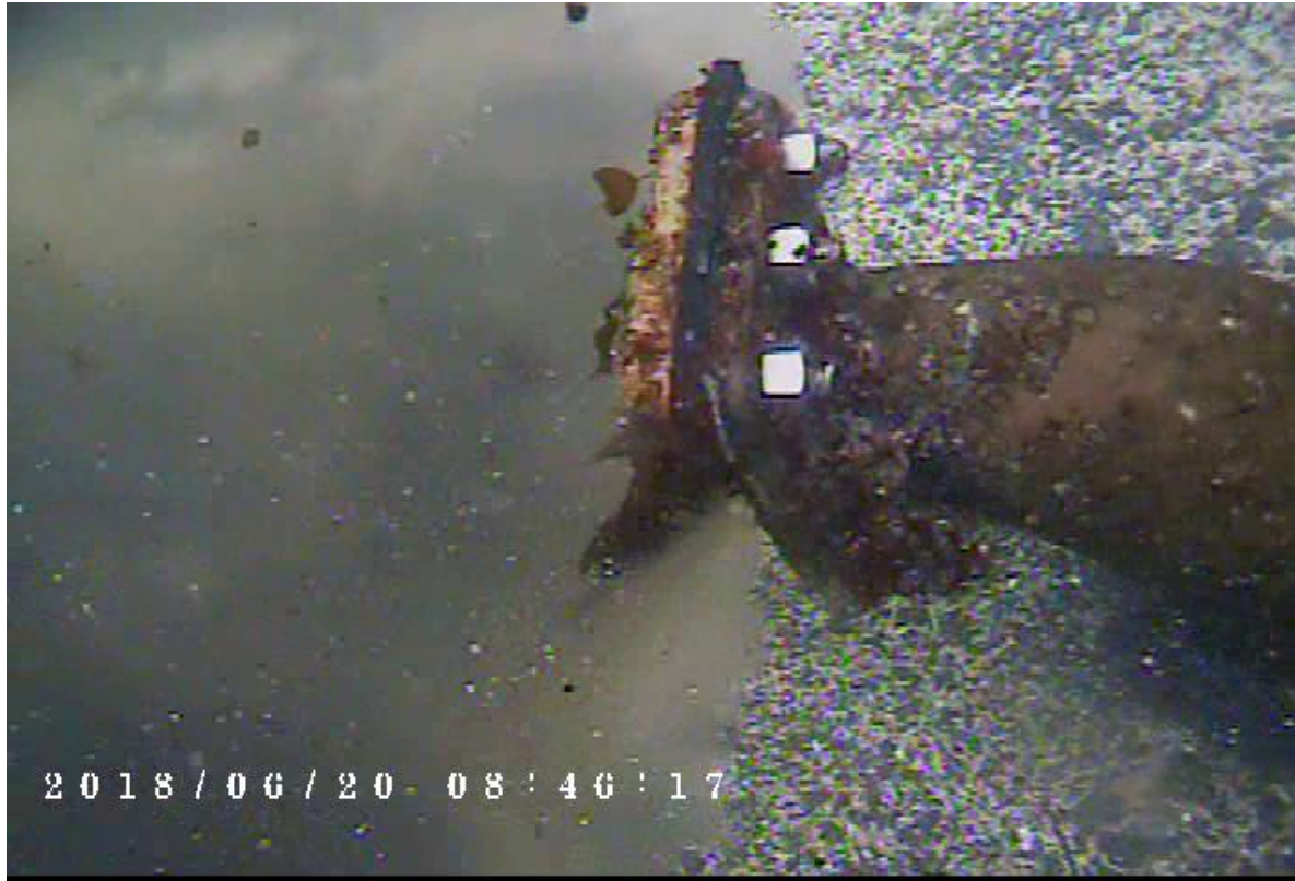
Photo 7 – Diffuser 7 showing strong flow
