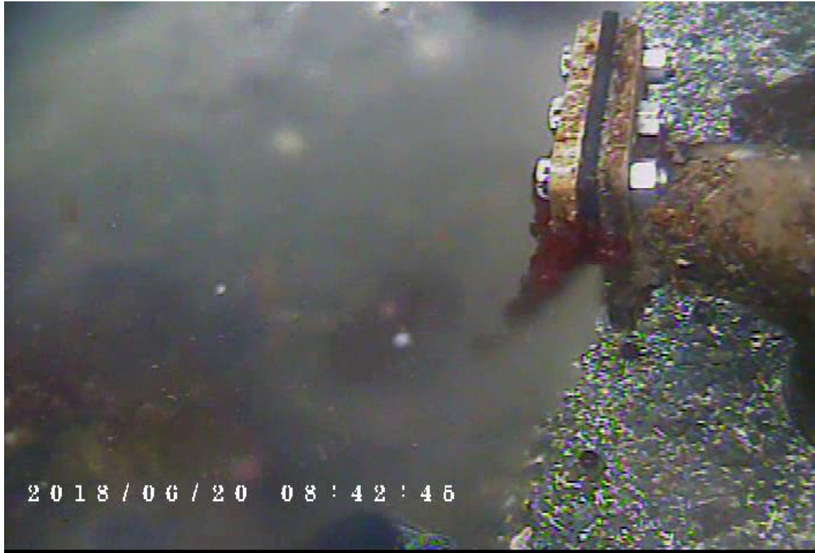
Photo 3 – Diffuser 3 showing strong flow
